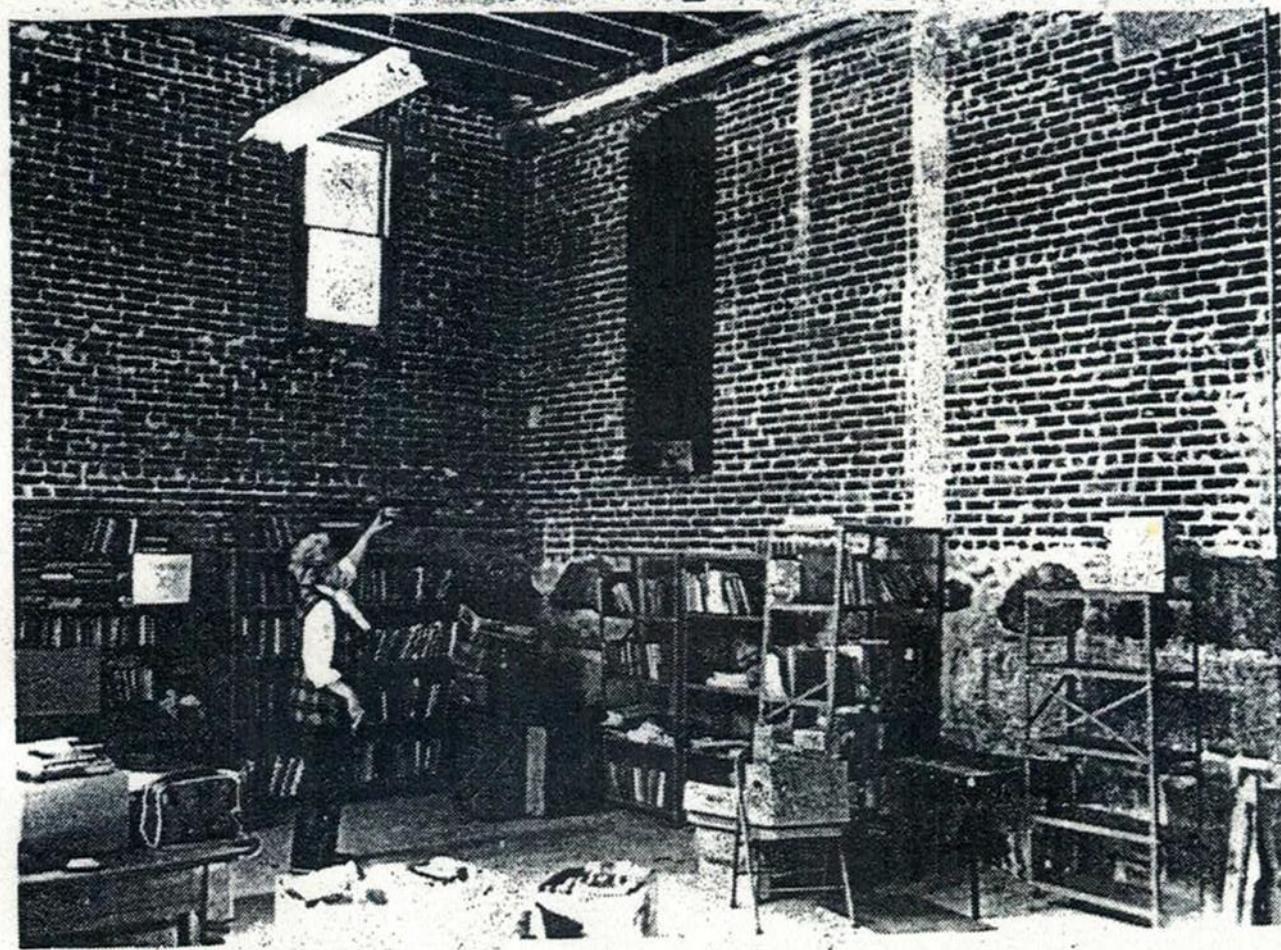
THAT'S WHERE the new floor is going. Helene Dermon indicates here where the new floor will be installed in the Tucker Free Library.
