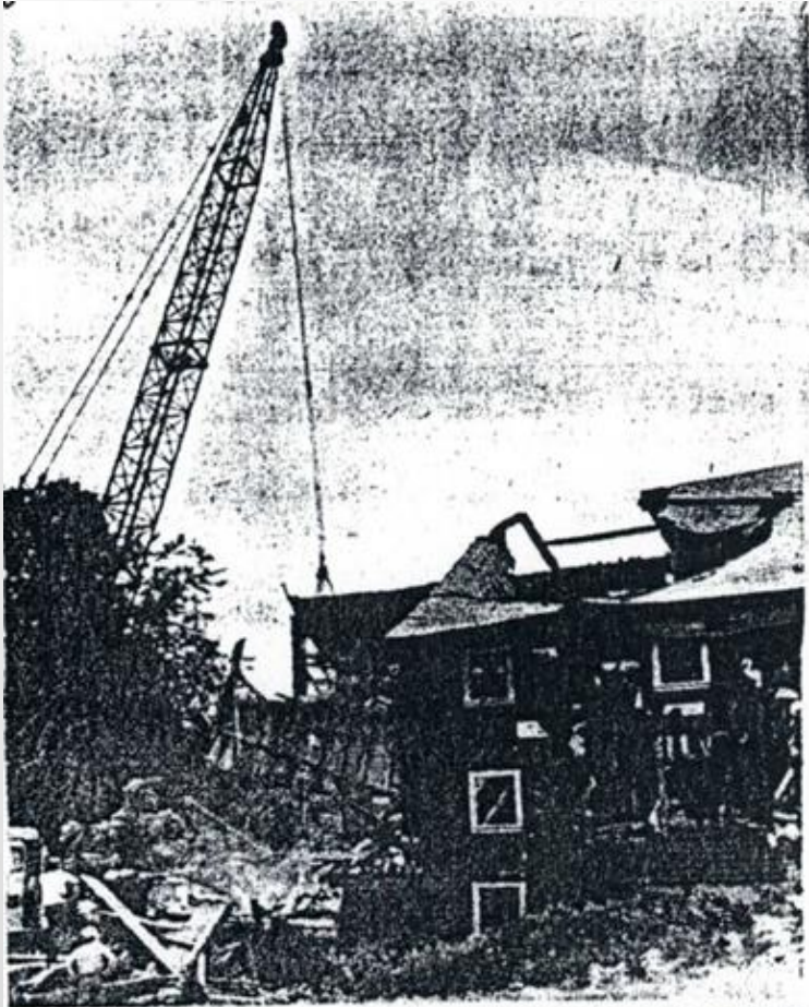
Calvin Tucker and George Sanborn help direct operations of the gigantic crane belonging to Ronald Garrison as it wrecks the 200 year old barn belonging to Merele Patenaude, beams of which will be used in the Francis Lane Childs Historical Room.
