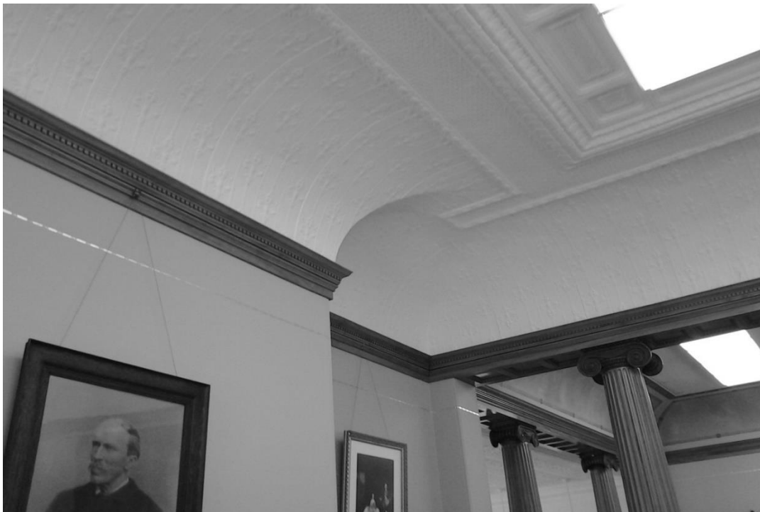
Image 41, Ceiling details of the NH Room. George Tucker's photo in the foreground, facing south west, photo taken: 1/31/13.
