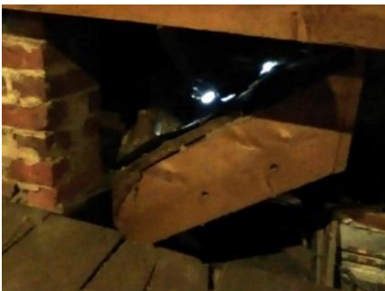
Image 98, Daylight at chimney flashing
