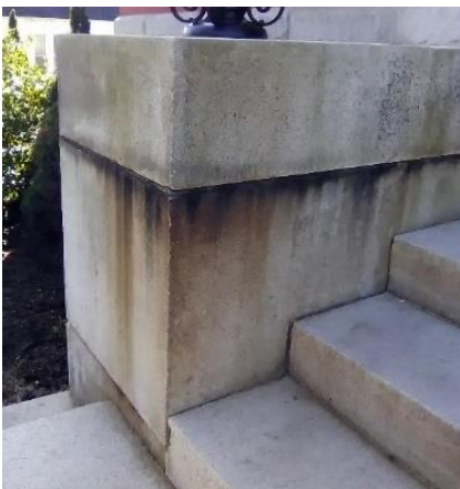
Image 77, Stone staining at entry
