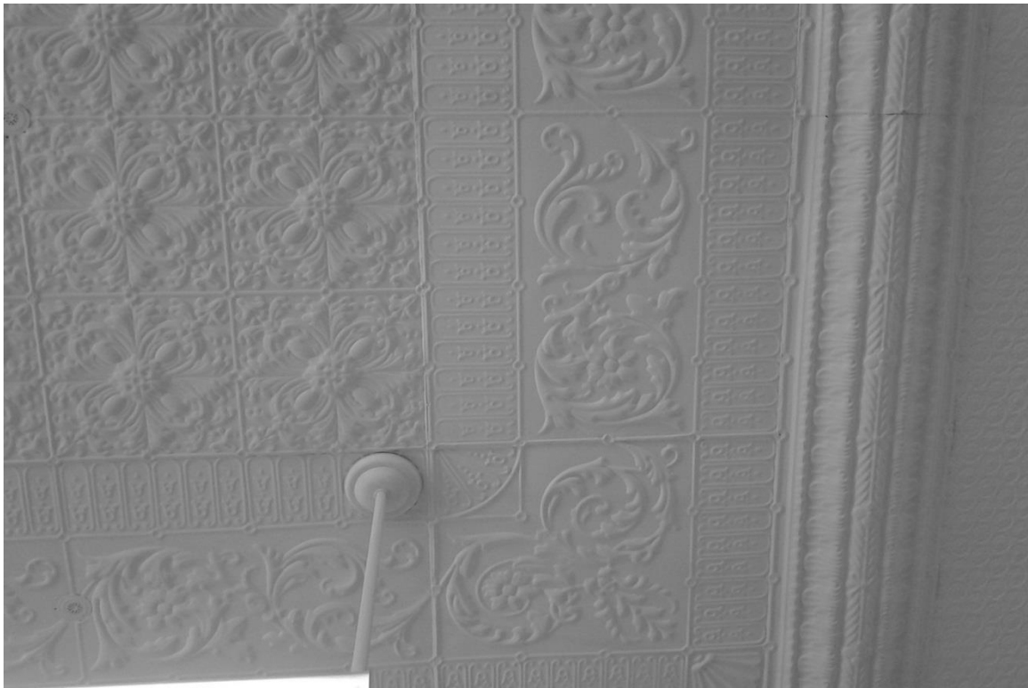
Image 44, Intricate tin ceiling details in the stack area, facing west, photo taken: 1/31/13.
