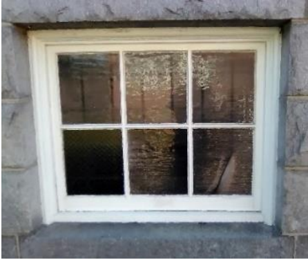
Image 87, Damaged and mixed glazing
