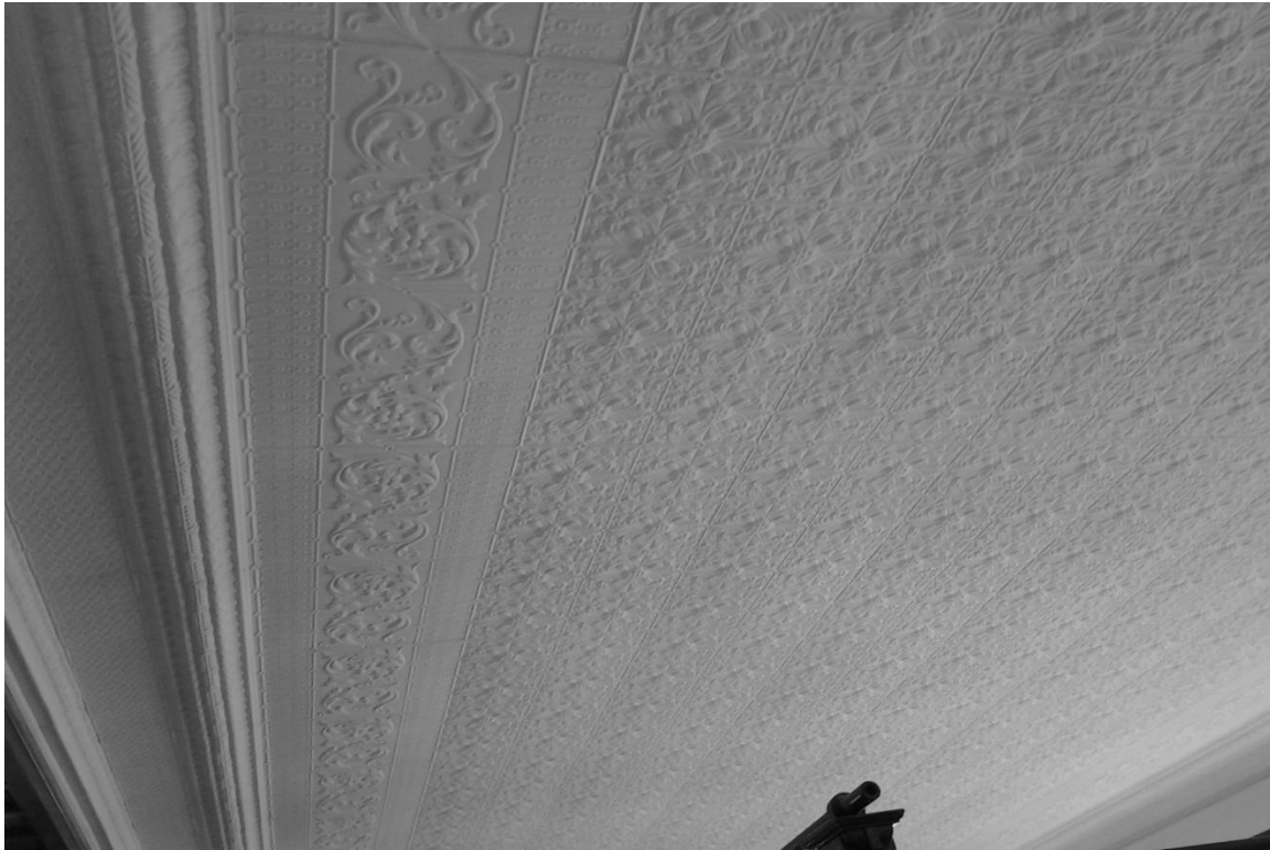
Image 42, Intricate tin ceiling details in the stack area, facing north, photo taken: 1/31/13.
