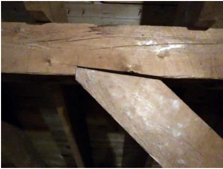
Image 96, Gap at truss
