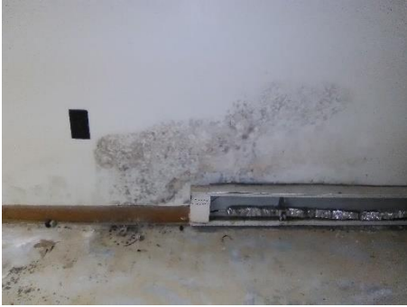
Image 88, Mold at Sub-basement
