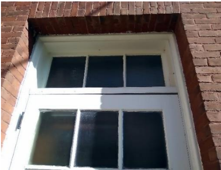
Image 83, Gap at J-Room Door
