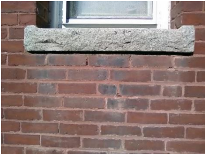
Image 76, Efflorescence below granite sills
