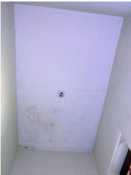
Image 95, Water staining at bathroom
