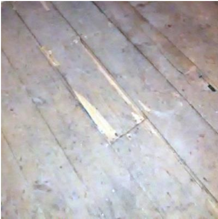
Image 97, Minor damage at Floorboards
