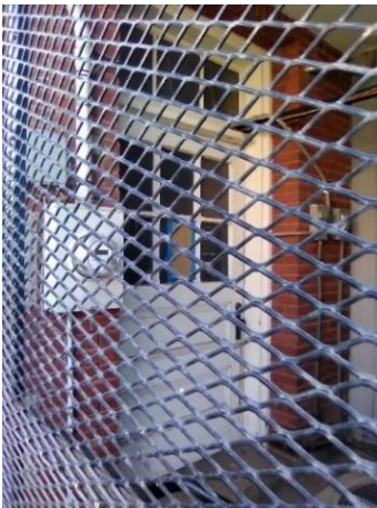
Image 86, Missing glazing boiler room door
